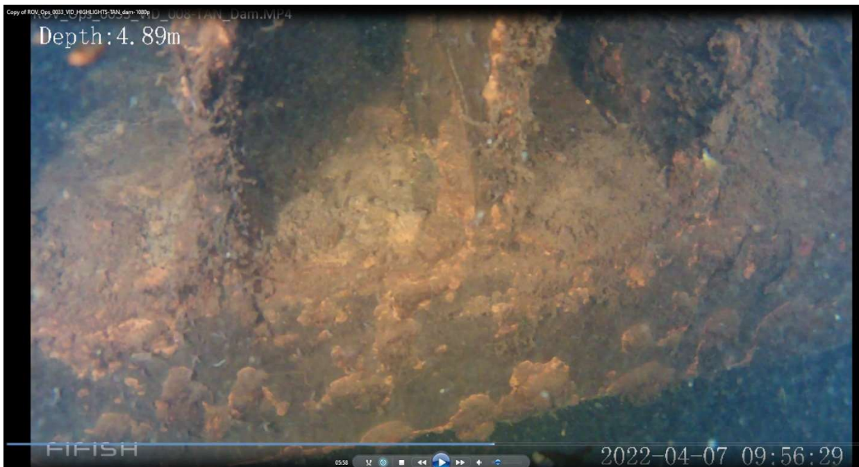
Figure 10: Example of biofouling accumulating on the surface of the existing Tantangara ROW coarse screens
