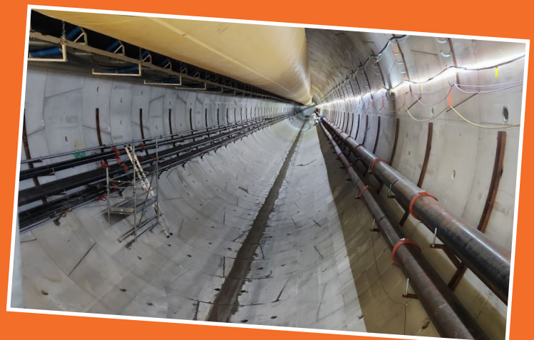
Above: Headrace tunnel being excavated by TBM Florence Left: Connection tunnel breakthrough at Tantangara
