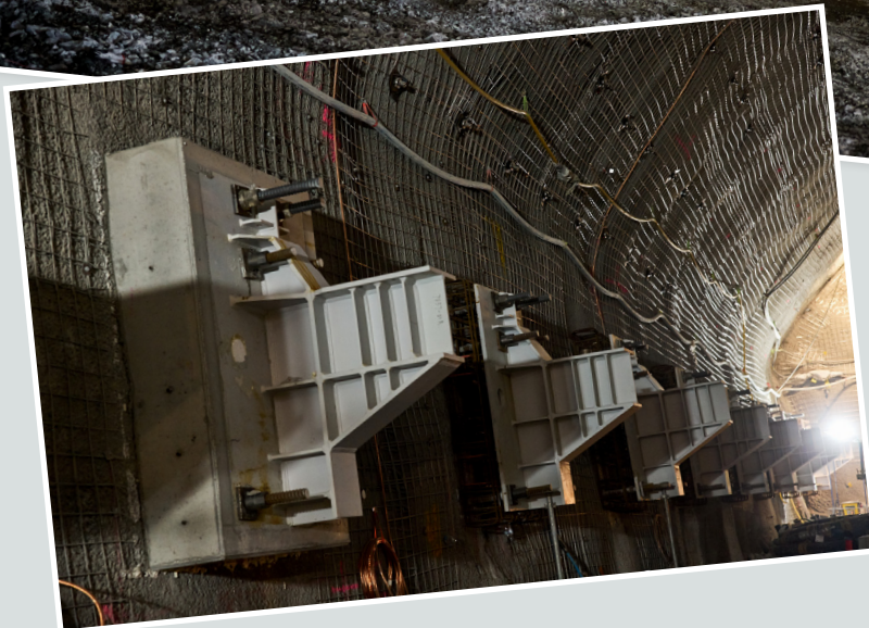
Left: Monitoring flora and fauna Above: Inside the power station caverns; corbels installed for construction cranes
