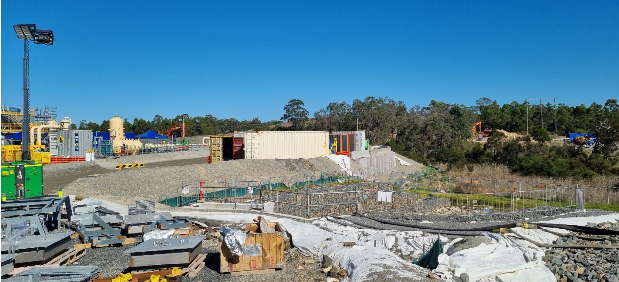
Photograph 6 - Site Water Discharge Infrastructure
